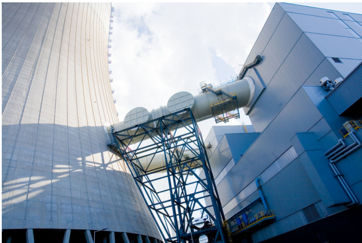
Photo showing the flue gas ducts adapted for the need of the CCP (flue gas pick up and return). Lower in the photo part of the cooling water installation for the CCP.
