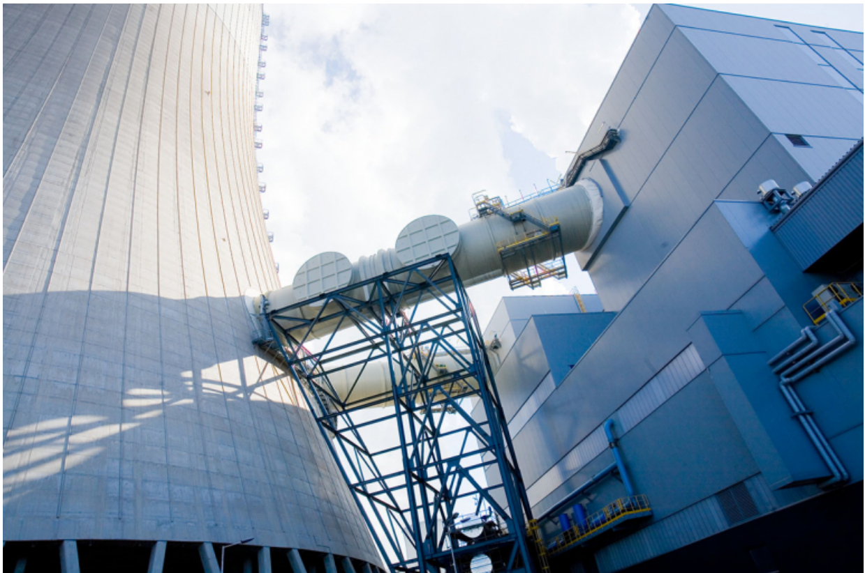
Photo showing the flue gas ducts adapted for the need of the CCP (flue gas pick up and return). Lower in the photo part of the cooling water installation for the CCP.
